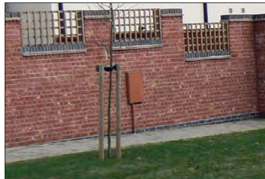
A meter box positioned on a rear boundary wall to an internal parking court and colour coded to the brickwork
