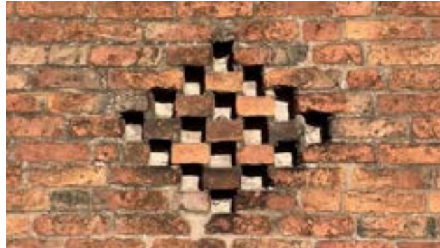
Figure 49: Traditional diamond shaped recessed brick features seen within barn walls along High Street.
