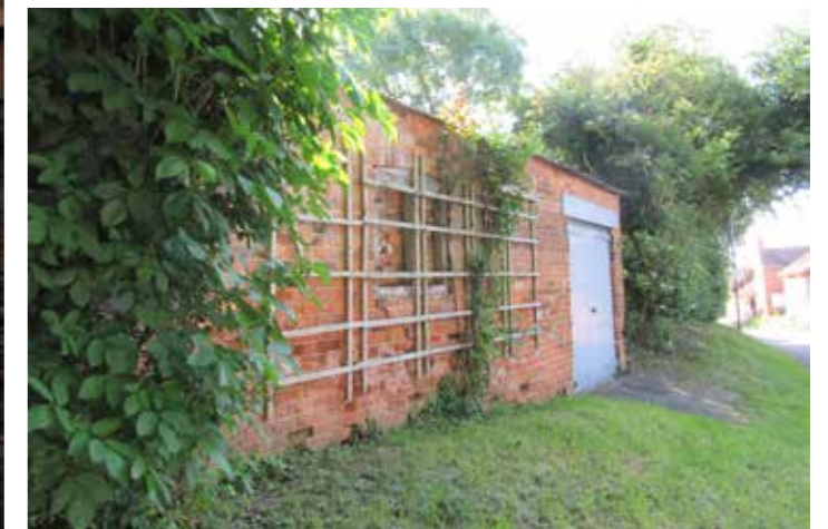
Fig 227 - 228: The old smithy building is a small yet distinct feature along Church Street, which has been well maintained and appears to be used for storage / ancillary residential purposes.
