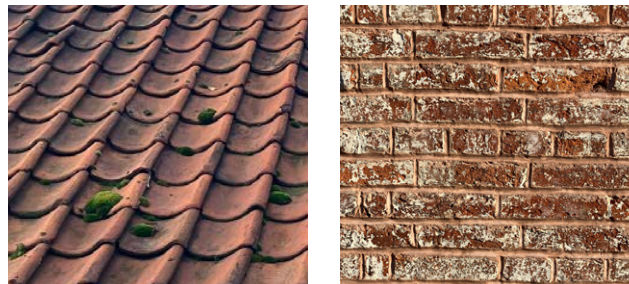
Figure 52: Typical character features seen across historic buildings in Elkesley include red pantiles, red brick, dentil brickwork detailing along the eaves, and dormer windows.
