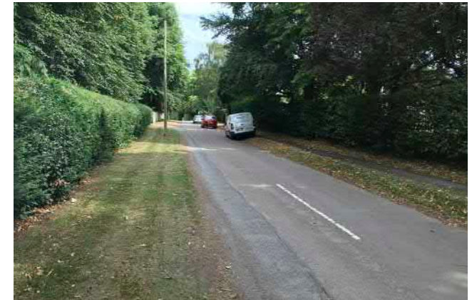
Paving along one side of Little Top Lane with hedge boundaries and wide grass verges.
