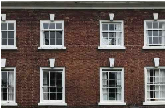
The Hall. Georgian recessed multi-paned sash windows which reduce in height at each storey. Window surrounds include a flat arch with a painted key stone and sill, and brickwork in a decorative Flemish bond.
