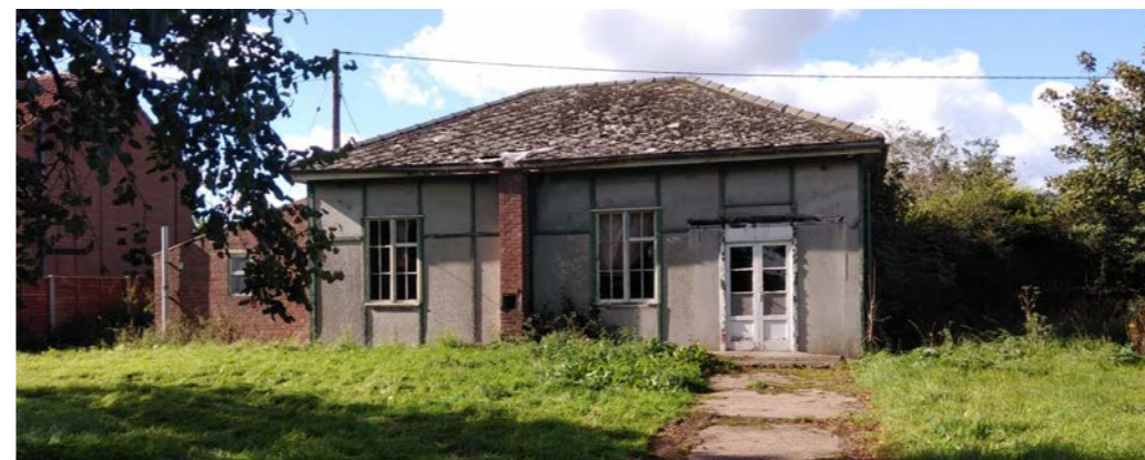
Fig 65: The derelict old village hall (now demolished) represents a local opportunity site.
