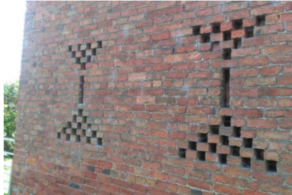
Fig 41: Red brick dominates the village townscape, particularly along Town Street, with some of the older farm buildings displaying particularly handsome brickwork and detailing, such as that seen in this image, where intricately arranged voids allow for air circulation into the building.
