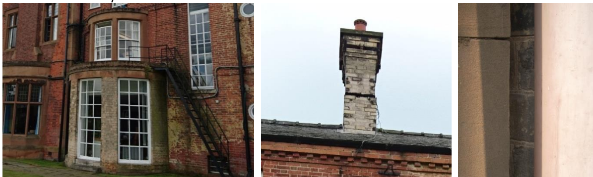
Yellow brickwork on rounded bay, chimney stack and in gap between bay and later extension.
